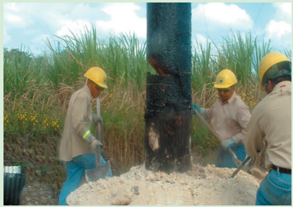
Employees working to repair a damaged pole from an act of sabotage.
